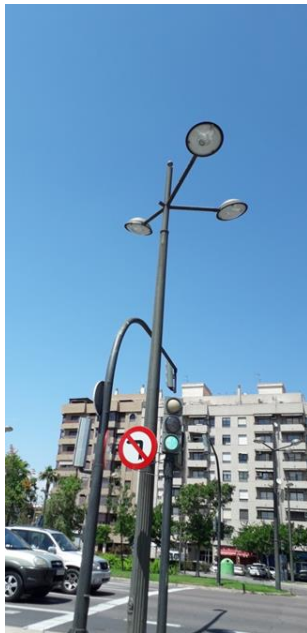
Street light spherical Campanar new LED - Valencia
